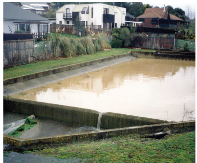
Figure 6-17: First generation stormwater systems, called silt traps, have a limited ability to treat stormwater and are very utilitarian in structure; making them unacceptable in today’s standards. Penruddock Rise silt trap.
