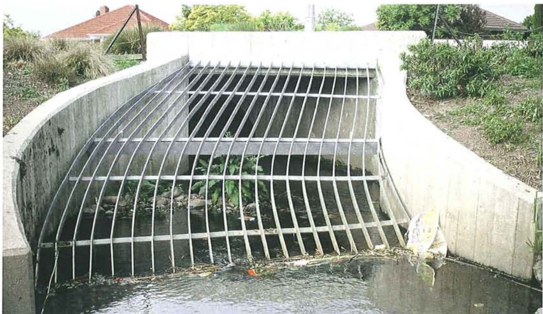
Figure 13-14: Slope has greatly increased this grill's surface area, enabling extra trapping ability during floods, and allowing for easy cleaning. Curvature significantly enhances the grill's appearance in this high visibility urban location. Dudley Creek grill at the corner of Ranger Street and McFaddens Road.
