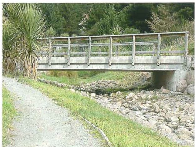
Figure 13-10: Bridges over hill waterways should have at least a 150 mm freeboard where large debris are expected. Glenstrae Stream at Drayton Reserve.
