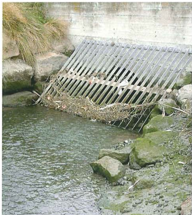
Figure 13-15: The firm stream base and shallow water allows cleaning of this grill from below while standing in the stream. The top edge of the grill rests on hooks allowing simple removal of the grill. Steamwharf Stream grill over the culvert at Ferry Road.
