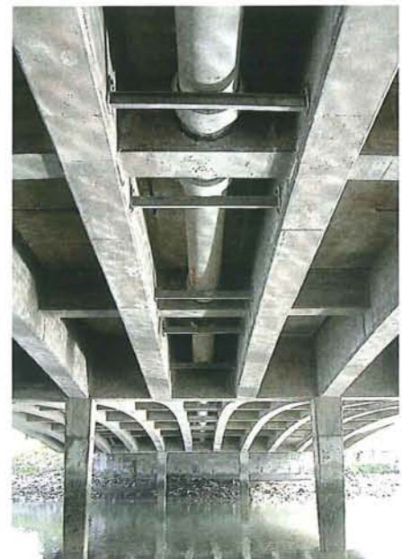
Figure 13-6: Attaching cables and pipes to bridge parapets is not acceptable. All such structures should be incorporated unobtrusively within the bridge structure (as illustrated). Ferrymead Road bridge, over the Heathcote River/Ōpāwaho.
