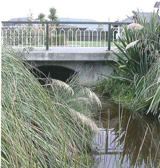
Figure 13-8: This culvert has been built to look like a bridge. As well a good appearance, this design ensures minimal constriction to flow and fish passage. Culvert over Corsers Stream at Brooker Avenue.
