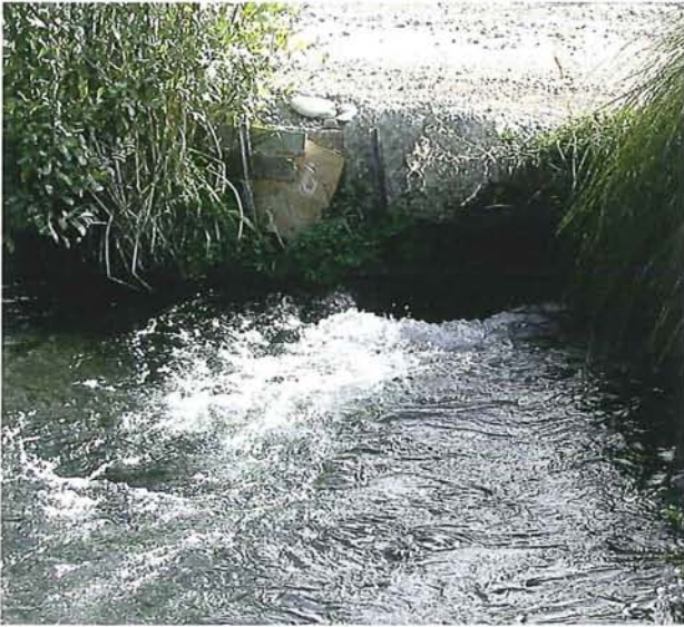
Figure 13-7: This culvert is undersized for the waterway. The resulting flow would prevent the upstream migration of some fish. North Boundary Stream at Clearwater Resort.
